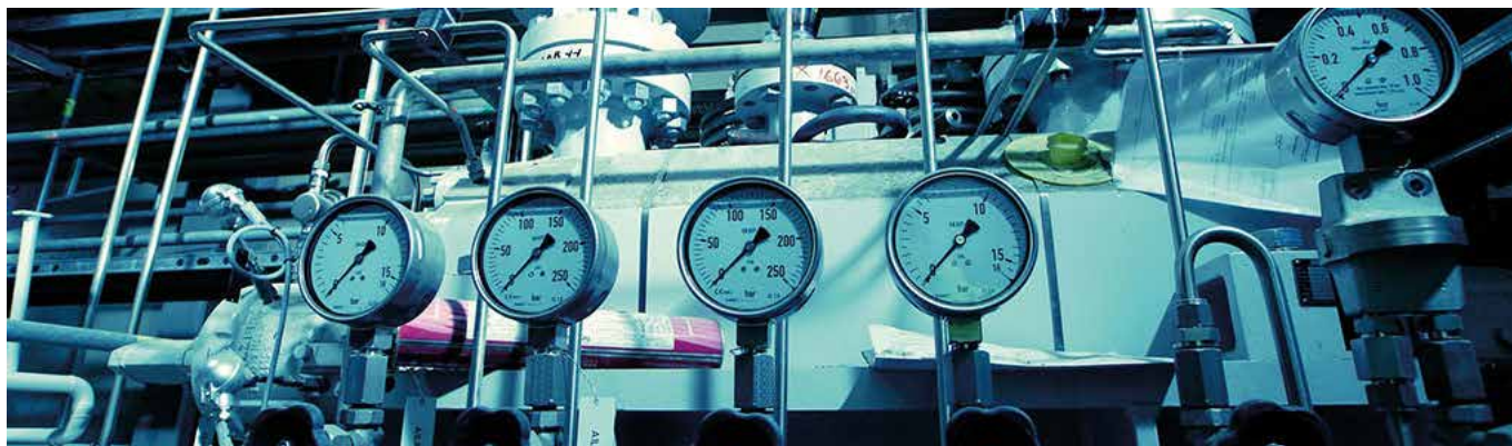
Steam pressure control systems
