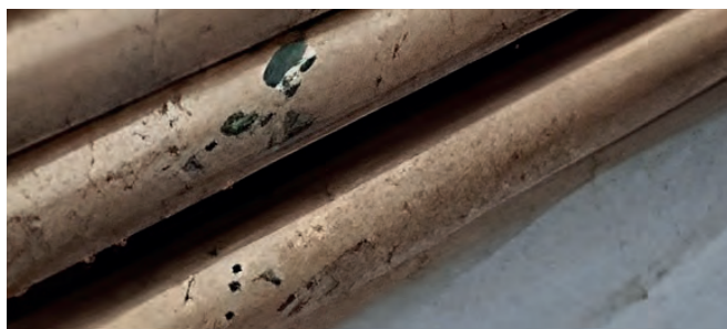
Figure 26 – Example of Pitting on Copper-Nickel Pipes
