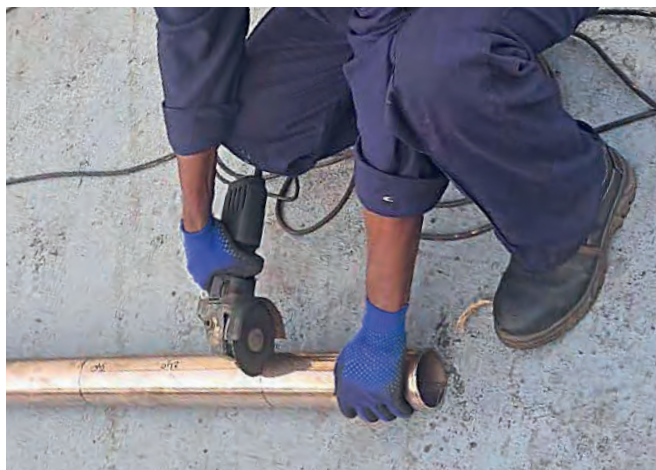
Figure 30 – Example of incorrect tooling
